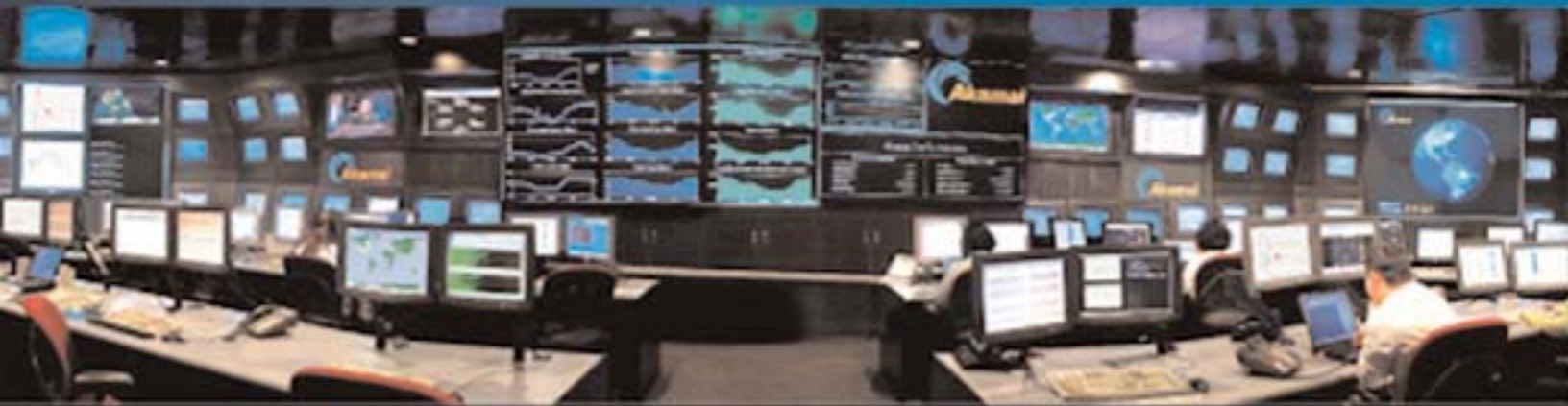
Akamai's Network Operations Command Center (NOCC)
